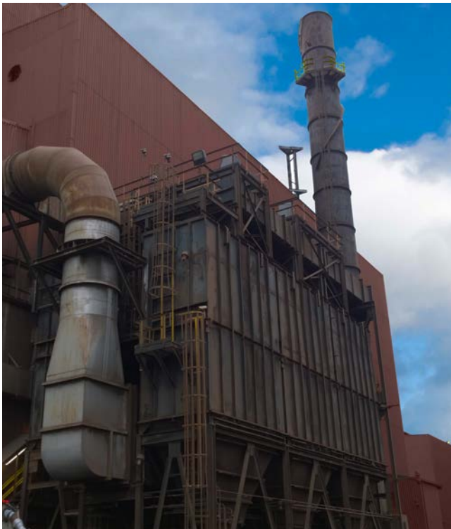
“Desulf” baghouse at a US steel mill. Leak analysis, pulse cleaning, DP, solenoids, valves, airflow, and temperature are monitored by an engineered B-PAC™ System (shown right).
