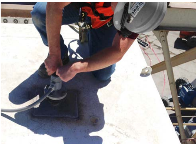
Auburn engineer commissioning particulate sensor.
