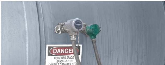
Installation of new DynaCHARGE™ particulate sensor (left) for filter leak detection by row.
