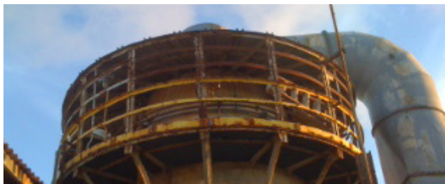
Acid discharge caused by baghouse upset conditions resulted in damage to process equipment structure.
