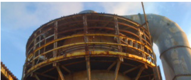
Acid discharge caused by baghouse upset conditions resulted in damage to process equipment structure.
