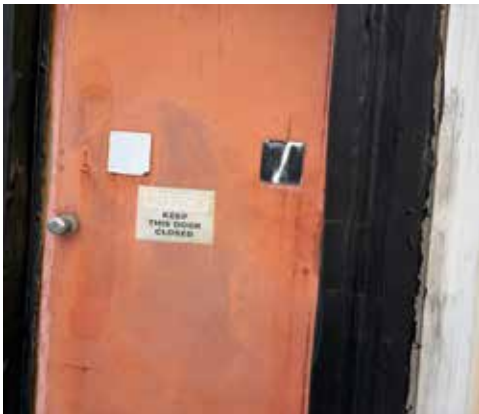
Tight door sealing is critical to containing airborne lead dust and protecting personnel from exposure.
